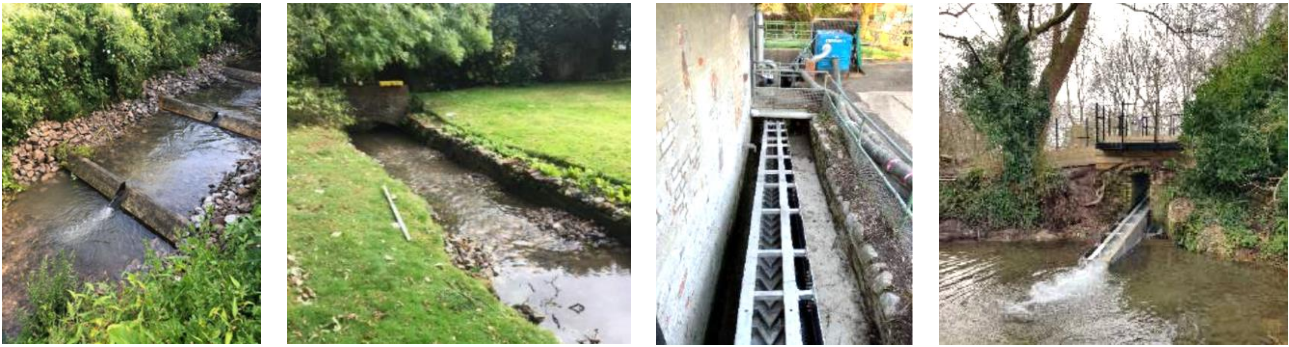
From left to right: Wellington Road Culvert, Garden Weir, Carisbrooke Waterworks Pond and Carisbrooke Mill Pond
